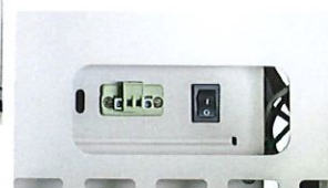
Remote Alarm contacts & Backup Battery Switch
